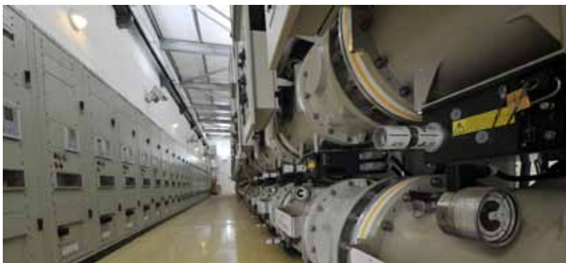
The City has invested significantly in Cape Town's electricity infrastructure
